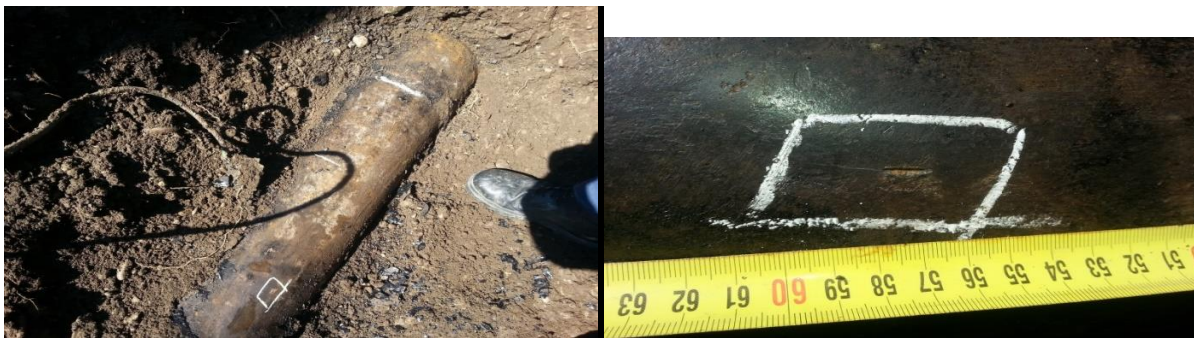
Image 4 - Rolling with extension to the outer surface 30 mm + corrosion (removed)
