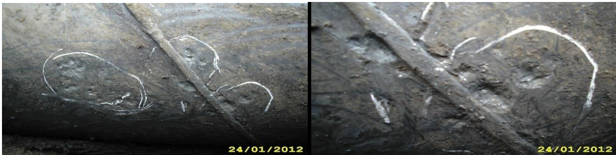
Image 6 - Generalized corrosion with helical bead damage (removed by replacement)
