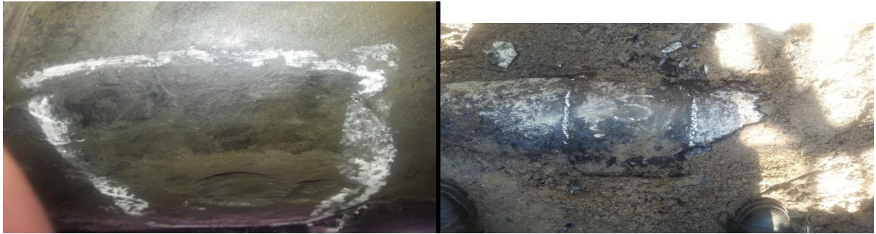
Image 2 - Pitting insulated in the lower part (6 o'clock), apparently good insulation (brittle with light mechanical action)
